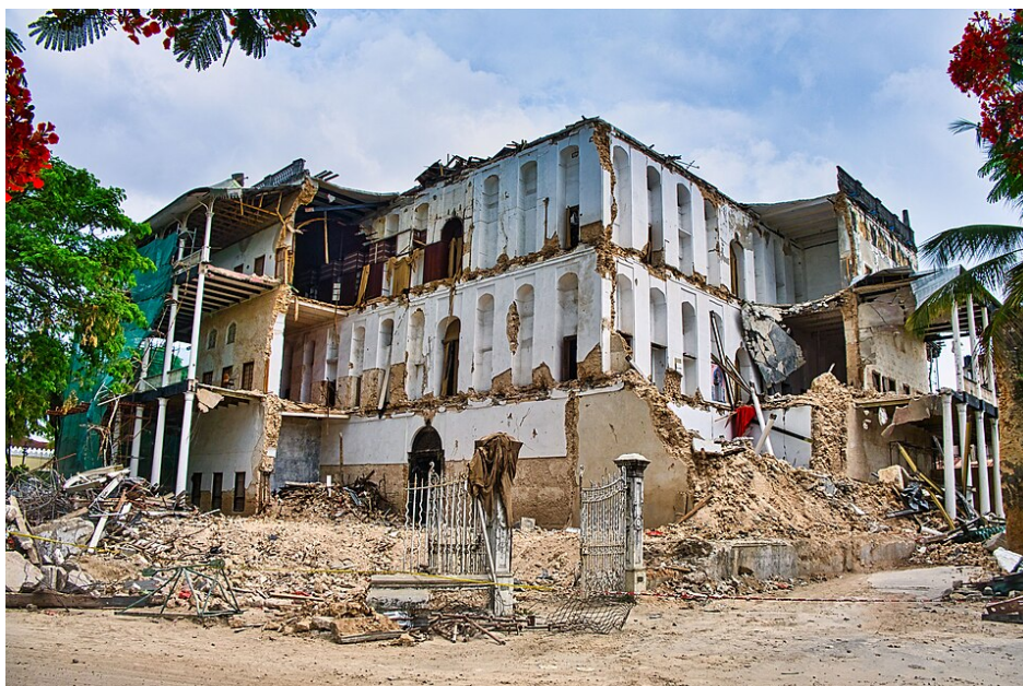
Figure 2. Structural damage at the House of Wonders (Beit al-Ajaib), Stone Town, Zanzibar, 2021. Photograph by Smartcam, Wikimedia Commons, CC BY-SA 4.0
